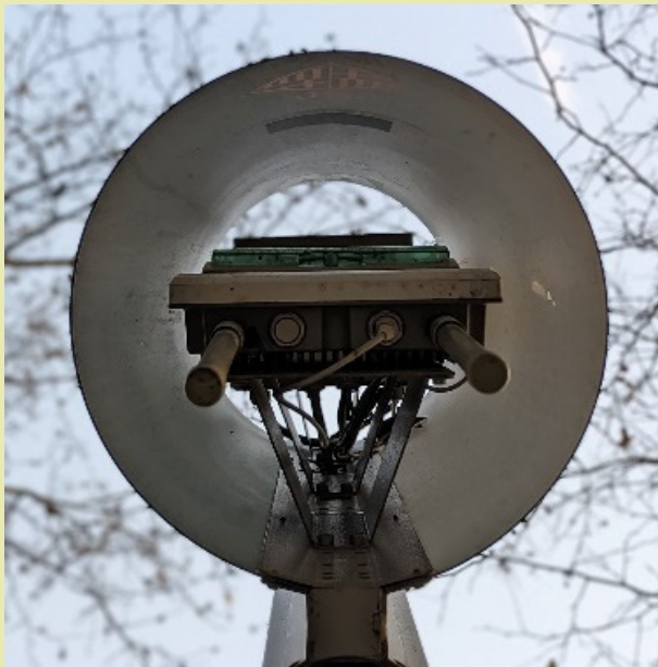
Intelligenter Mast in Barcelona
