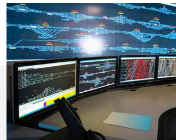
Digital Train Control System
