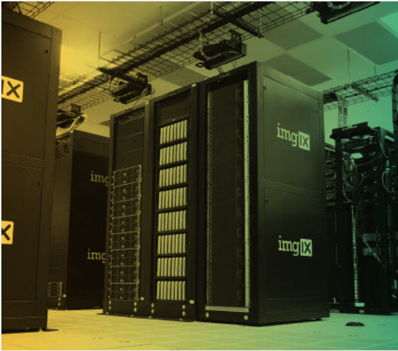
Image: Data centre, imgix
