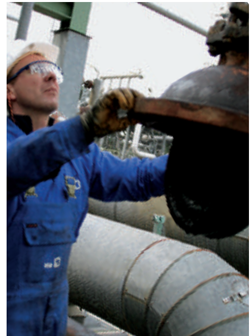
Meeting the deadline: major valve rehabilitation projects, like this one in a refinery near Karlsruhe / Germany, often require KSB service teams to be on site for several weeks on end.
