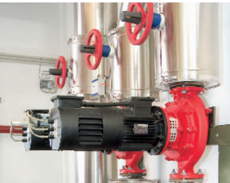
Built-in energy efficiency: the power input of variable speed pumps is matched to actual requirements.
