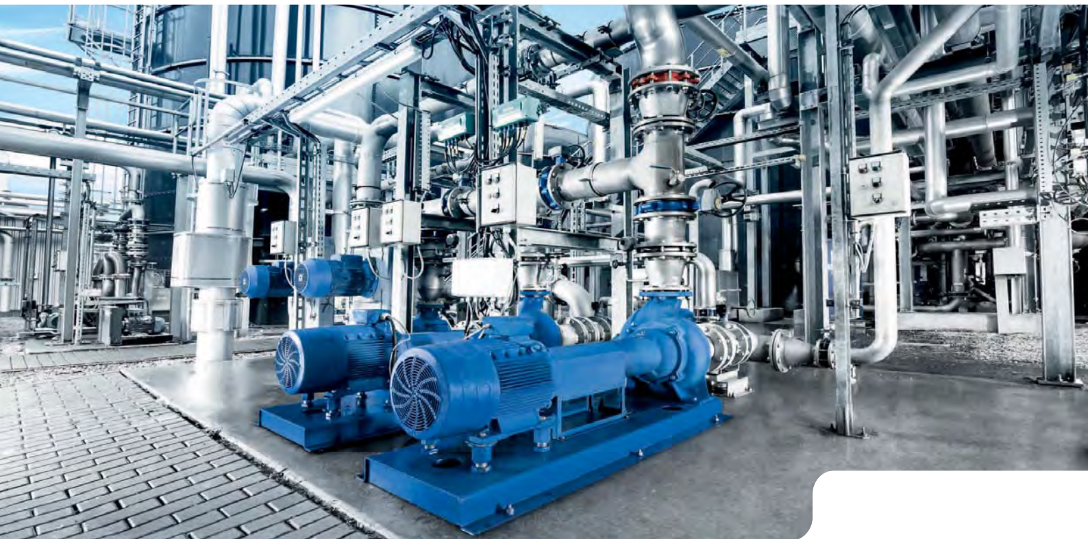
High-performance components: Sewatec® volute casing pumps and Isoria® butterfly valves used in a bioethanol plant.
