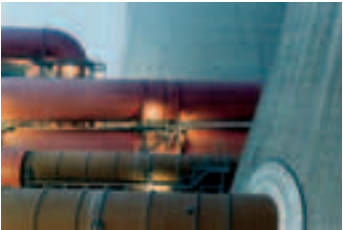
Purified gas lines leading to cooling towers
