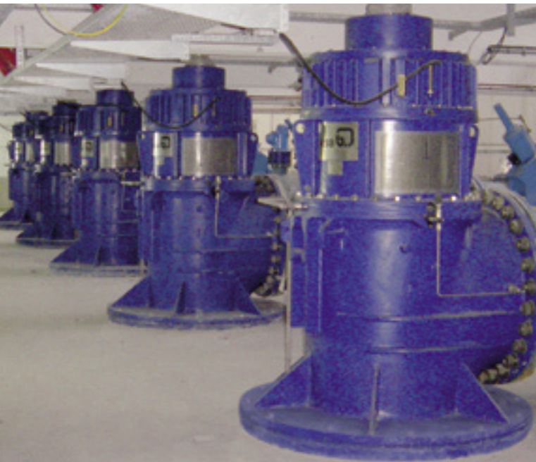
In a new pumping station for Istanbul's drinking water supply system, six KSB tubular casing pumps transport 43,000 cubic metres of water per hour.
