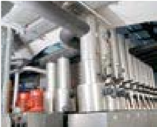
The air-conditioning system of the „Berliner Bogen“ office building in Hamburg is equipped with KSB pumps and valves.
