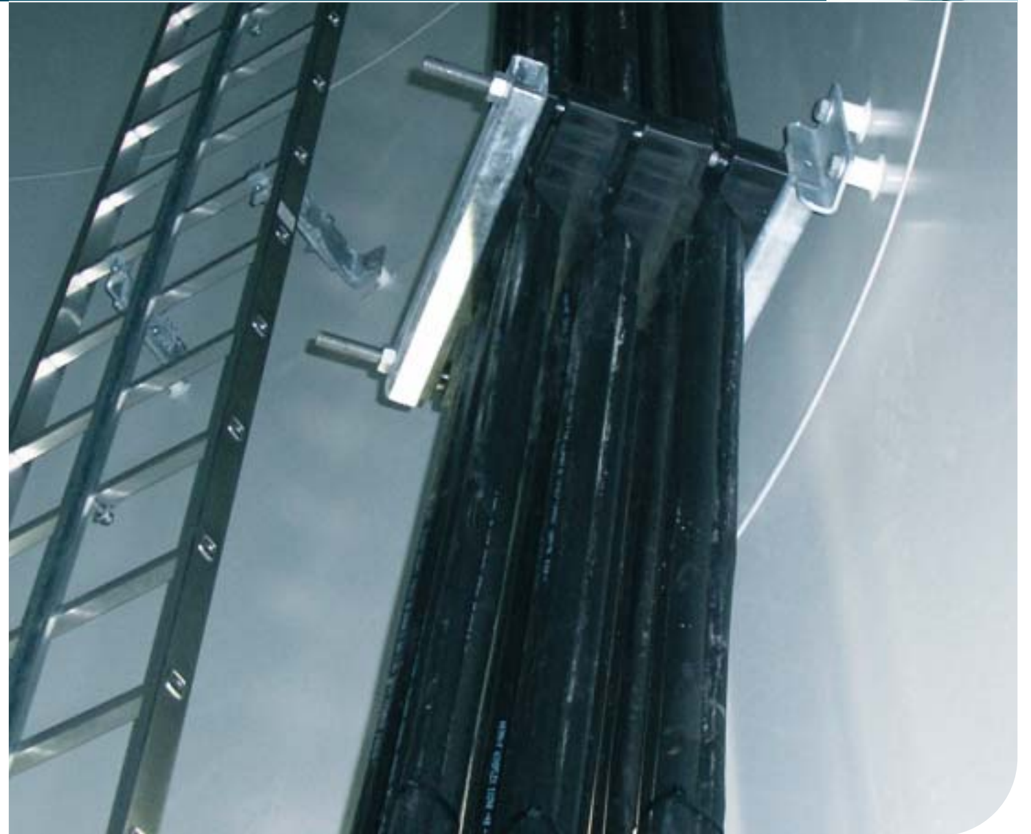
Regulated rise cabling in a turbine tower.
