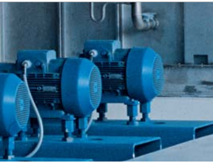
Volute casing pumps of the Etanorm series in the heating supply system of an industrial plant
